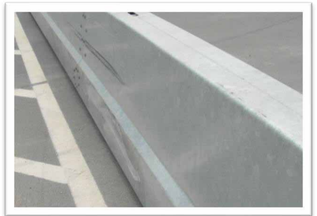
Typical Impact Damage
