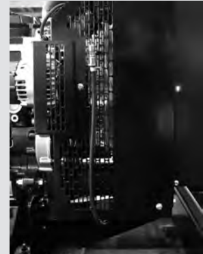
Coolant Drain tap
