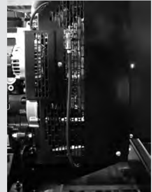
Coolant Drain tap
