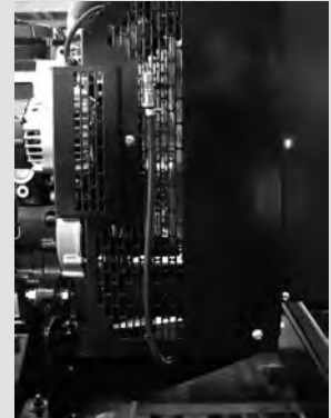
Coolant Drain tap
